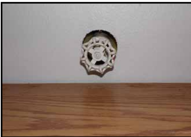
Main water shutoff in downstairs bathroom
