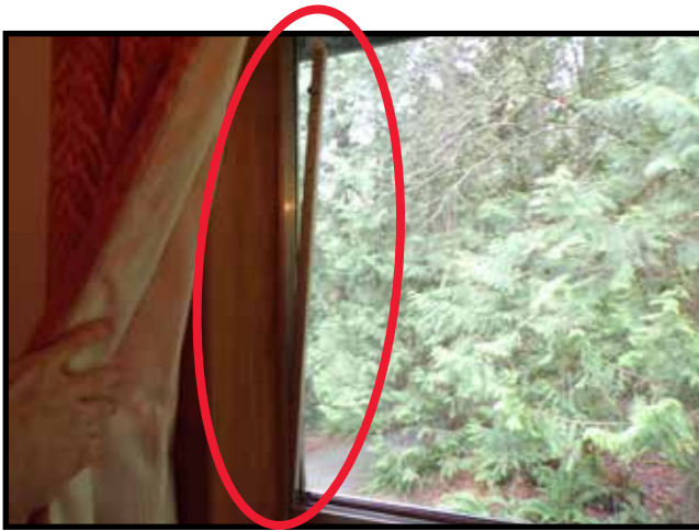
Broken balance on master bedroom window
