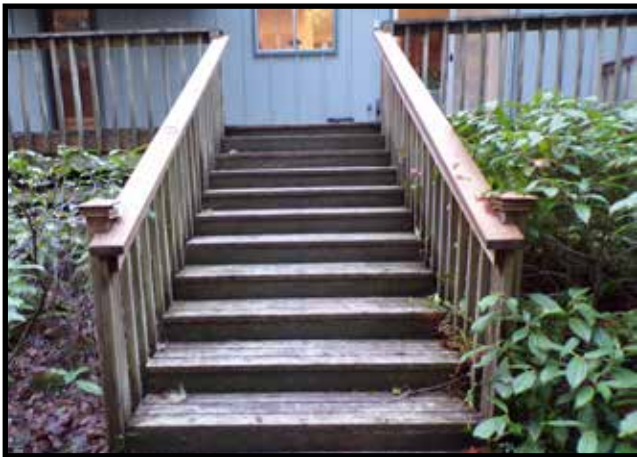
Deck stairs without proper handrail
