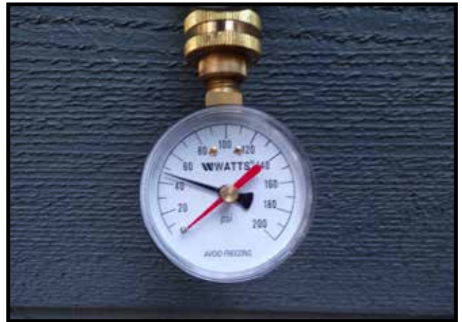
Water pressure reading of approx 48 psi
