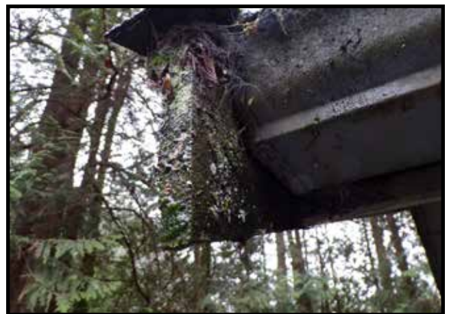
Signs of rot on garage fascia
