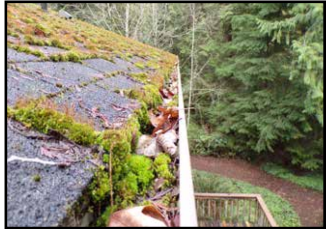
Clogged gutters on upper roof
